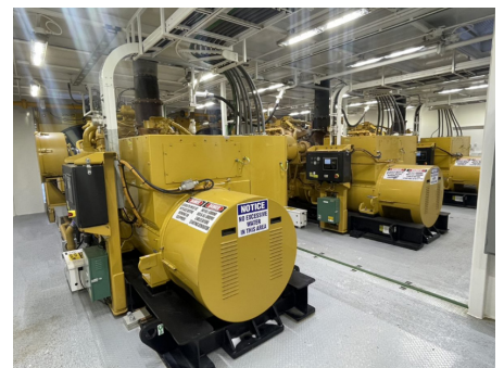
Figure 2: Inside of the Natural Gas Generator Building
