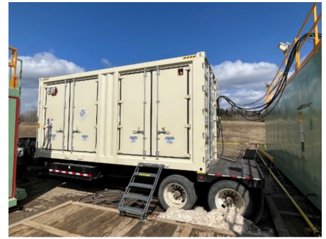
Figure 3: ESS Container and Trailer.
