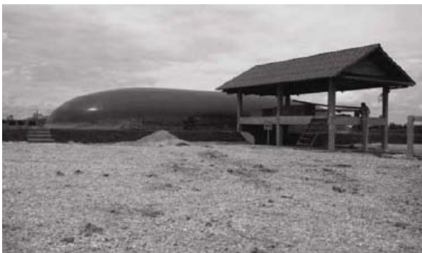
Figure 8: Buffer Tank and Digestion Process in Thailand
