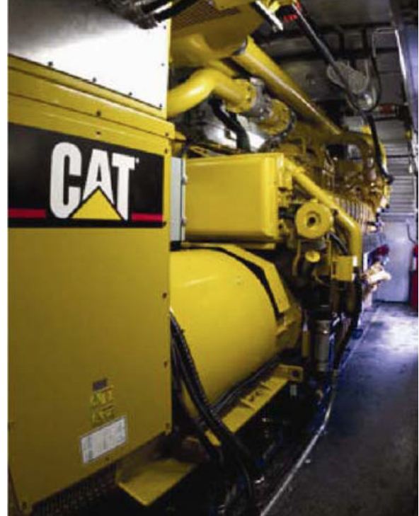
Figure 4: Landfill Gas Engine Generator Set
