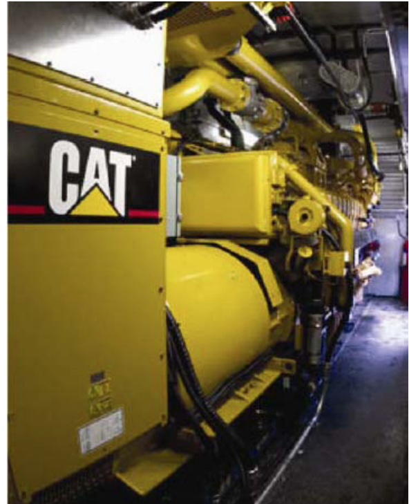
Figure 4: Landfill Gas Engine Generator Set
