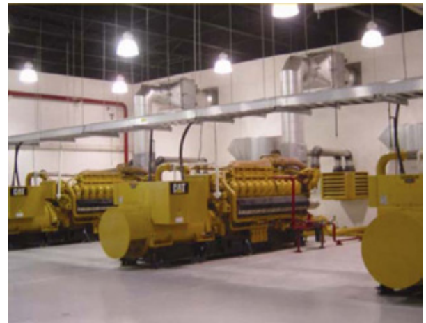
Figure 2: DG in Hurricane City Power Plant
