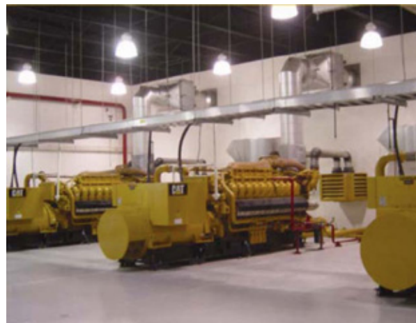
Figure 2: DG in Hurricane City Power Plant
